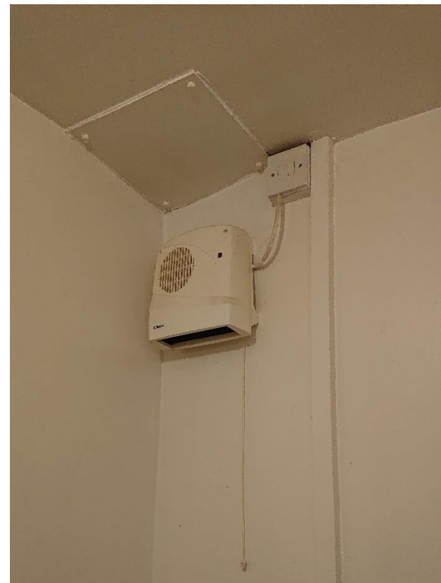
Inefficient fan heater in the kitchen
